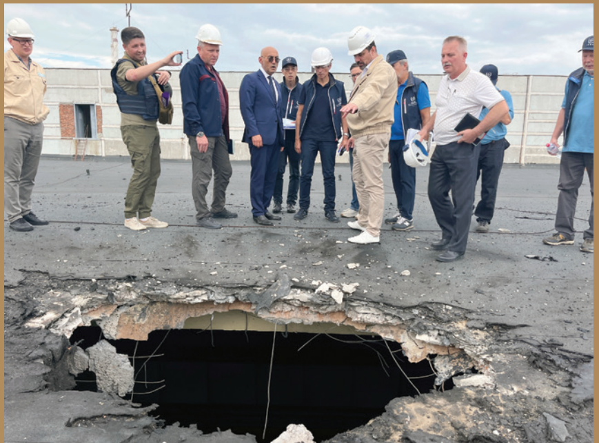
The IAEA team observes the damage caused by shelling on the roof of the special building at the ZNPP that houses, among other items, the fresh nuclear fuel and the solid radioactive waste storage facility. (Photo: IAEA)
