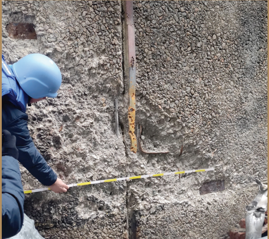
Wall of the Unit 4 reactor building at ZNPP after the shelling on 19–20 November 2022. (Photo: IAEA)
