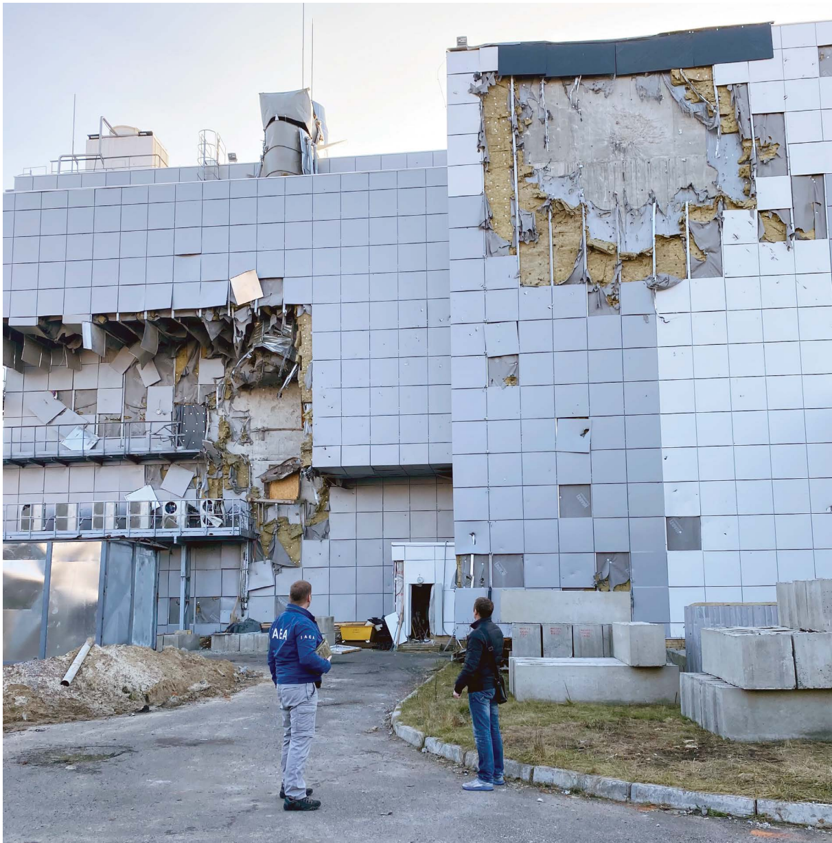
IAEA staff observe damage from a rocket attack at the KIPT subcritical assembly on 22 November 2022. (Photo: KIPT)
