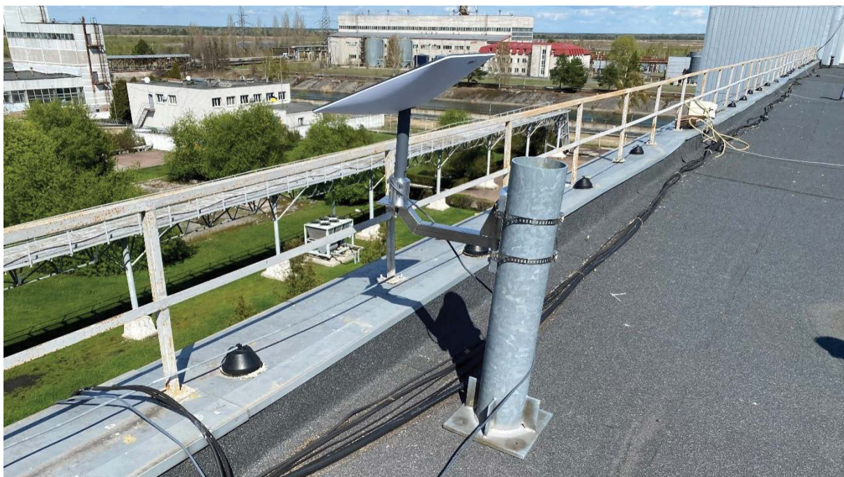
The new satellite communication system for RDT installed by the IAEA at the Chernobyl NPP, 27 April 2022. (Photo: IAEA)
